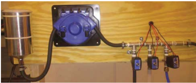
Figure 2: Mixing vessel, pump, and valves
